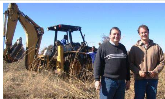
John Mixon and contractor, Jaco, smile as the backhoe breaks ground for the new Administration Building.
